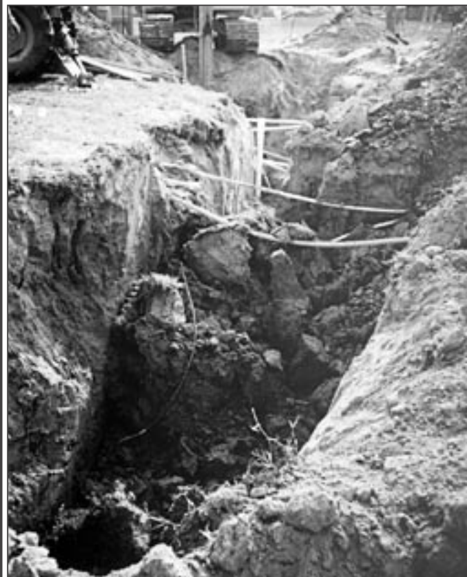
The workers in this trench were not so fortunate. Two men lost their lives here because sensible – and required – protection was not provided in the form of proper, life-saving shoring or shielding.
