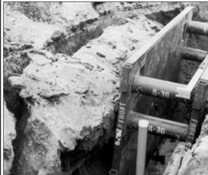
At least two people's lives were saved by this trench shield when a massive chunk of soil gave way, slamming the side of this trench box.
