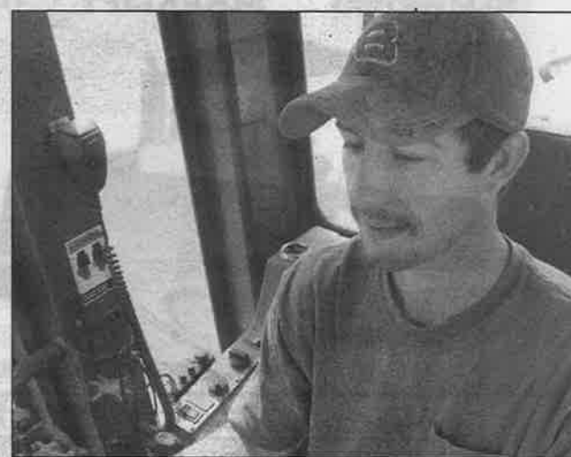
Lance Cox keeps an eye on the in-cab 3-D machine controller that allows precise cutting of slope on a baseball field in a large sports complex in Heber Springs, Ark.
