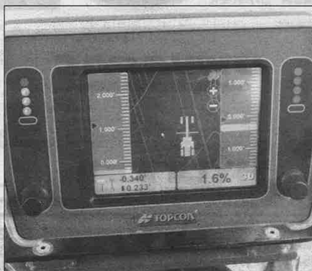
With 3-D machine control, an operator "sees" exactly where he or she is on a job via an in-cab controller.
