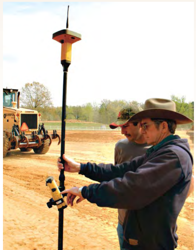
The Topcon Survey Rover allows Larry Cox to check grade anywhere on the site and perform layout work.
