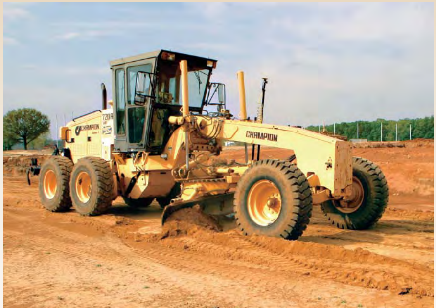
Cox Construction initially purchased a Topcon GR3 Base Station and Survey Rover to outfit their Champion Motor Grader for this project in Heber Springs, AR.
