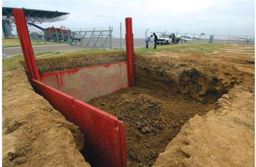
Slide rail systems such as this one, being installed in Memphis, are just one of several protective systems available to construction and utility companies and their contractors.
