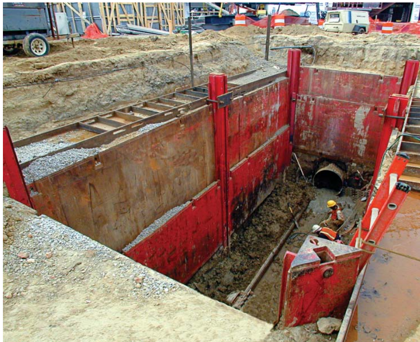
Often nearby surface structures, utilities, or underground installations make trench boxes the only sensible way to protect employees working below grade.
