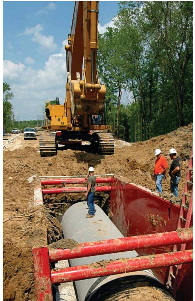
Adequate means of entrance and exit must be provided for workers, allowing them to exit trench boxes or shoring systems quickly. Note the ladder in the foreground to the right.
